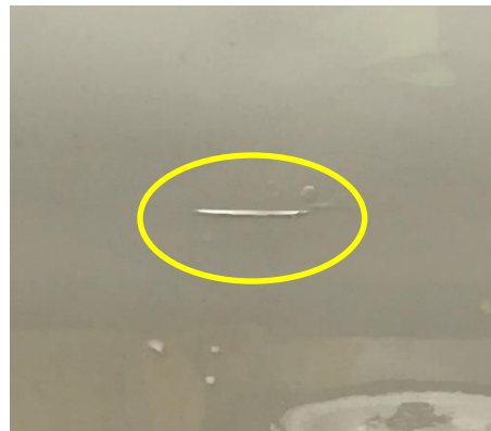
Close up image of ridge and protruding fastener head
