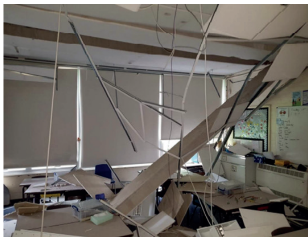
Photo source: LGA, RAAC Article 2023
