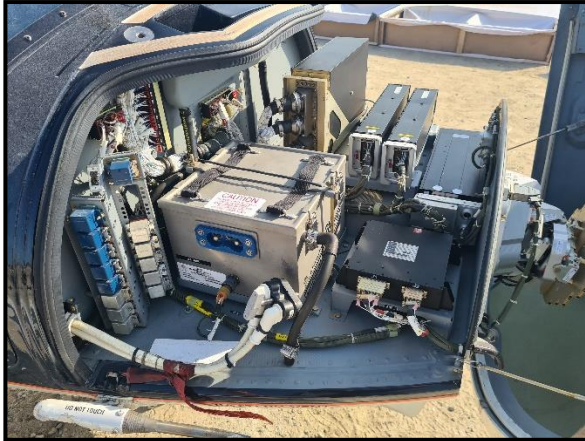
Overview of the avionics equipment
